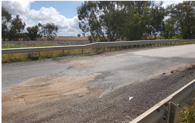
Canola Way failures at Cowabbie Creek
