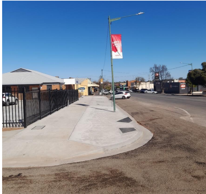
East Street kerb and footpath upgrade between Elwin Street and Watkins Lane
