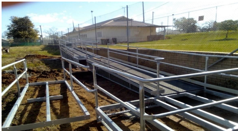
New accessible ramp to the lower courts – under construction – Narrandera Tennis Club.
