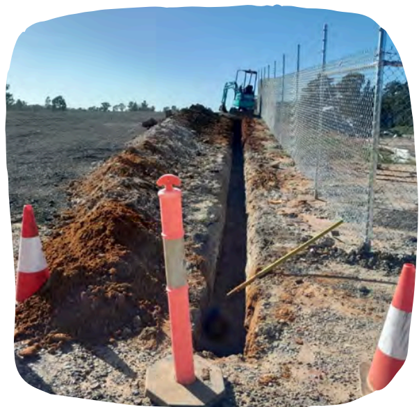
Fire service and fire hose reel installation Narrandera landfill
