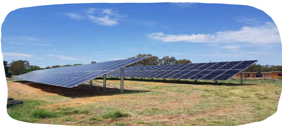
80.6kW ground mount system – Narrandera Sewer Treatment Plant
