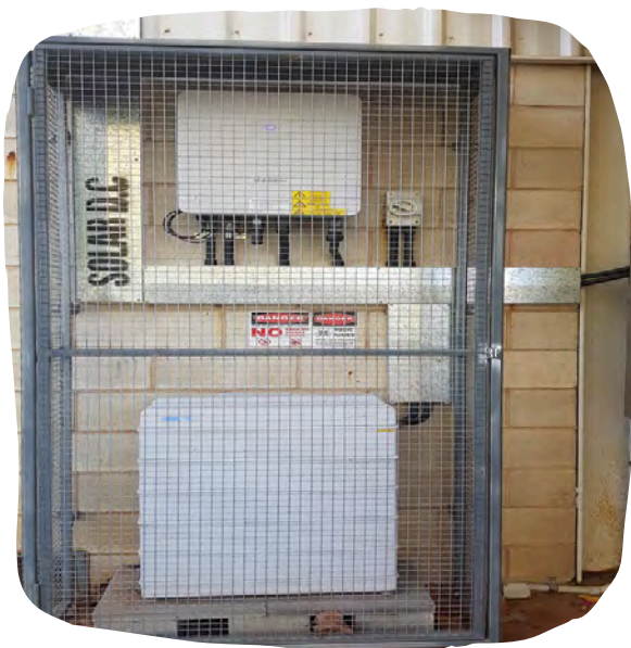
15.7kWh Battery storage – Narrandera Sports Stadium
