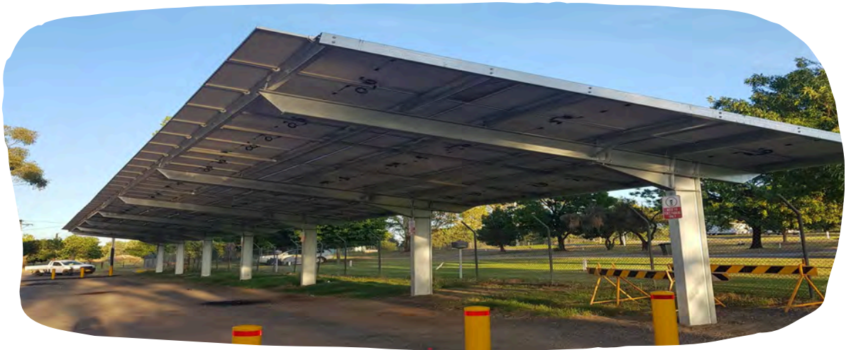
74.7kW Carport system view from the carpark – Lake Talbot Water Park
