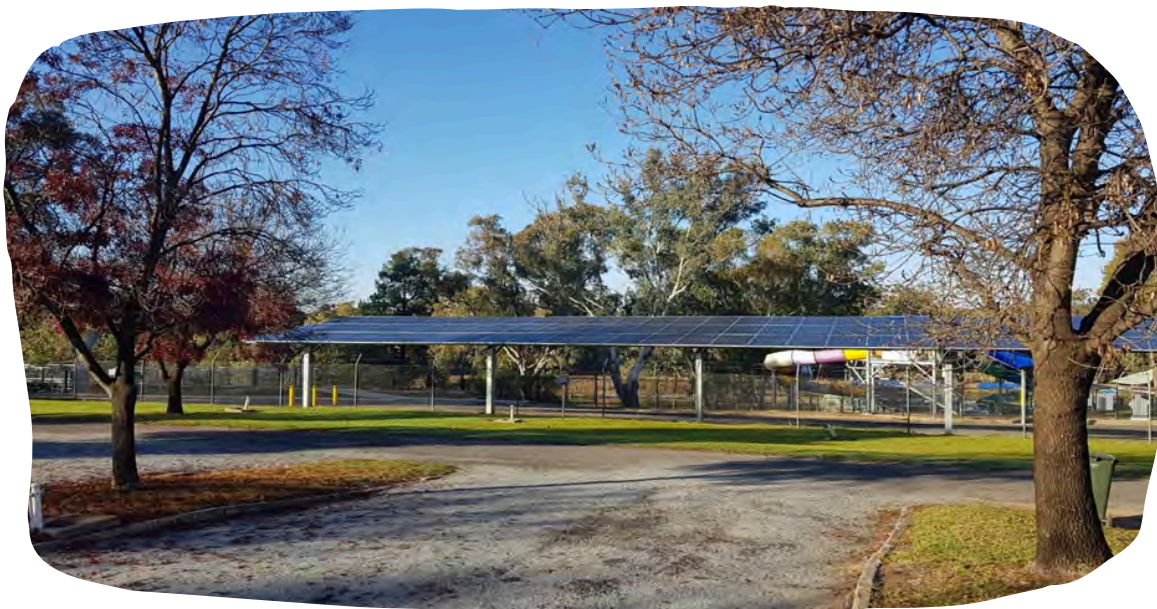
74.7kW Carport system view from the Caravan Park – Lake Talbot Water Park
