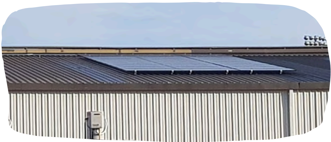
14.7kW roof mount system – Narrandera Sports Stadium
